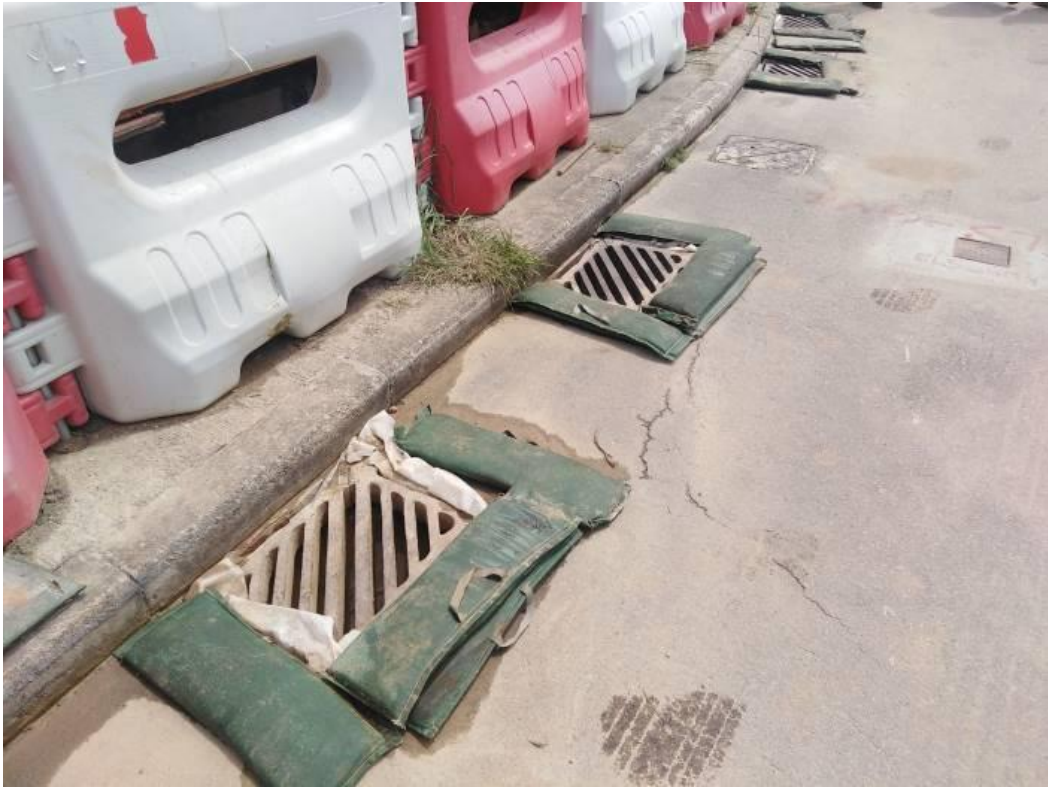
Date of site inspection: 24 August 2022 Gullies were bunded by sand bags to prevent surface runoff.
